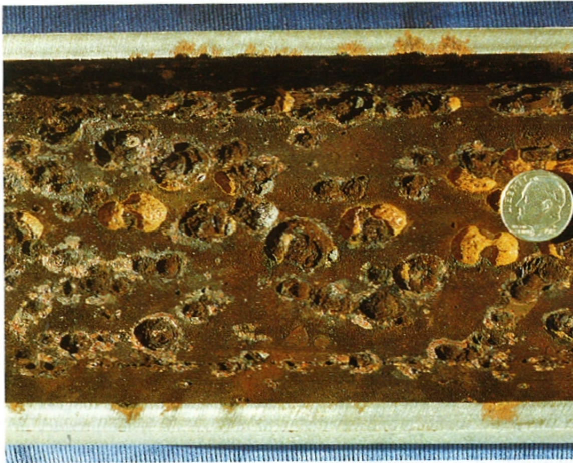
Figure 5.8 Heavily pitted surface of a mild steel cooling water return line. Note the deep localized metal loss surrounded by aureoles of rust. Pitting is common when oxygen concentration varies greatly over time.
