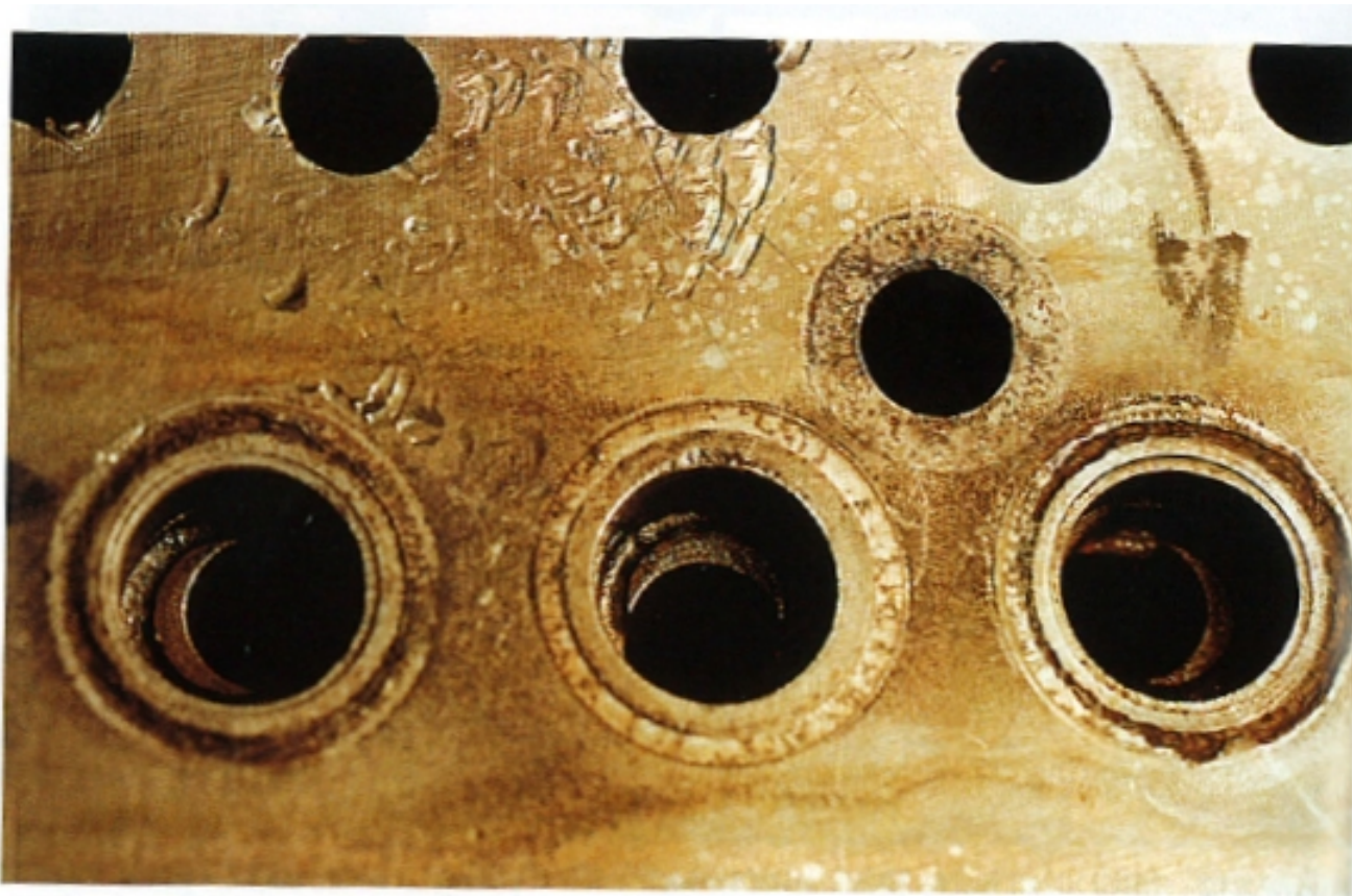
Figure 2.14 Close-up of annular regions below rubber O-rings on a cast iron valve block. Note how damage varies from hole to hole, probably due to variation in the crevice geometry.
