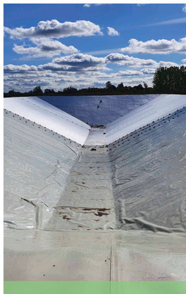
The heat pit storage is a pioneer project. The development project has received DKK 13 million from EUDP which is the supporting pool of the Danish Energy Agency for development projects.
