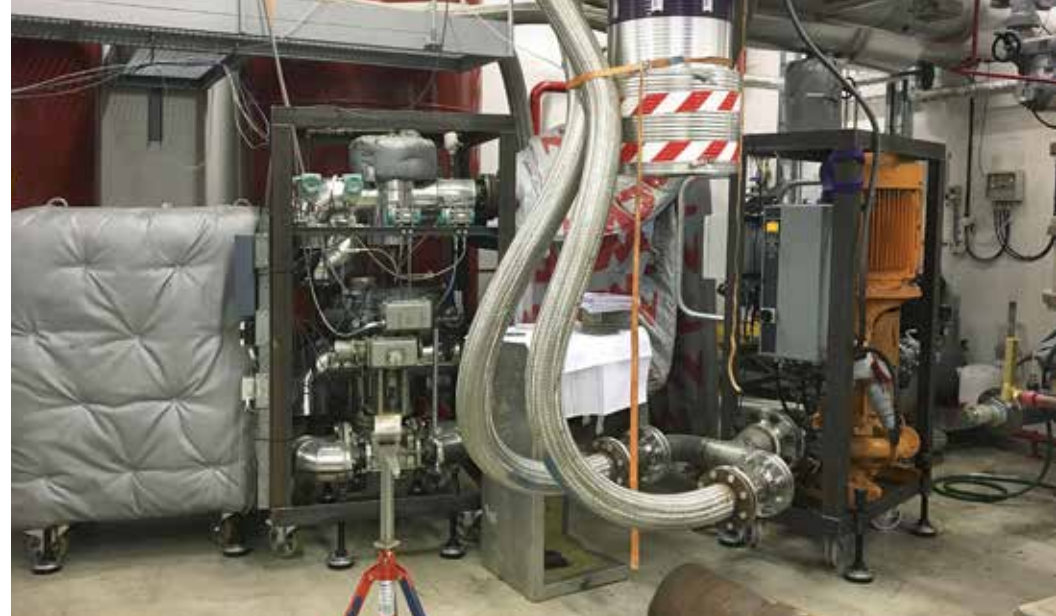
VEKS' "homemade" mobile exchanger also forms part of the preparedness. It functions as an alternative to the mobile boiler which is usually used when considerable and long-term servicing work is on the way. Several of the local district heating companies in VEKS' supply area have borrowed the boiler in connection with planned repairs.
