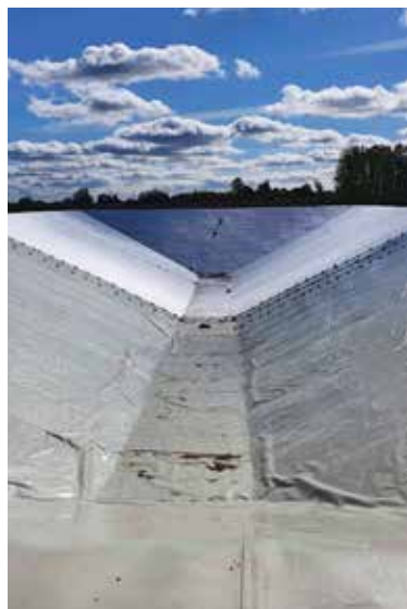
The heat pit storage is a pioneer project. The development project has received DKK 13 million from EUDP which is the supporting pool of the Danish Energy Agency for development projects.
